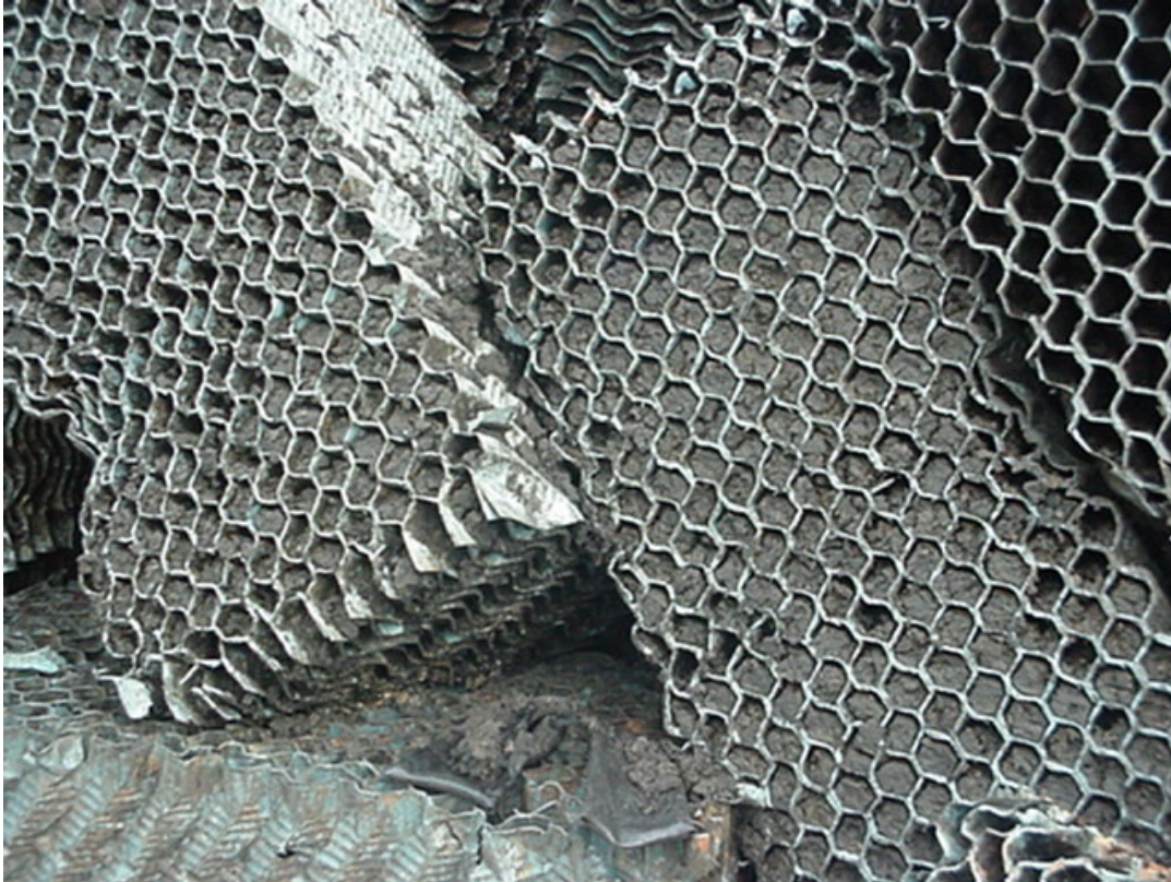
Figure 3 – Photo of Media Modules Removed from Anaerobic Reactor
