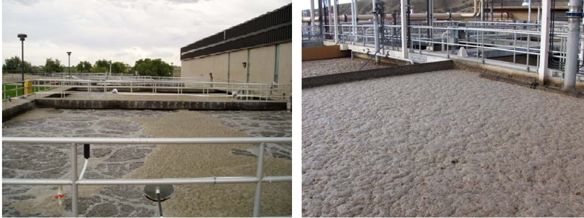
Figure 13. Typical surface foam at the Broomfield IFAS facility, and foaming during start-up at the Henry N. Wochholz IFAS facility
