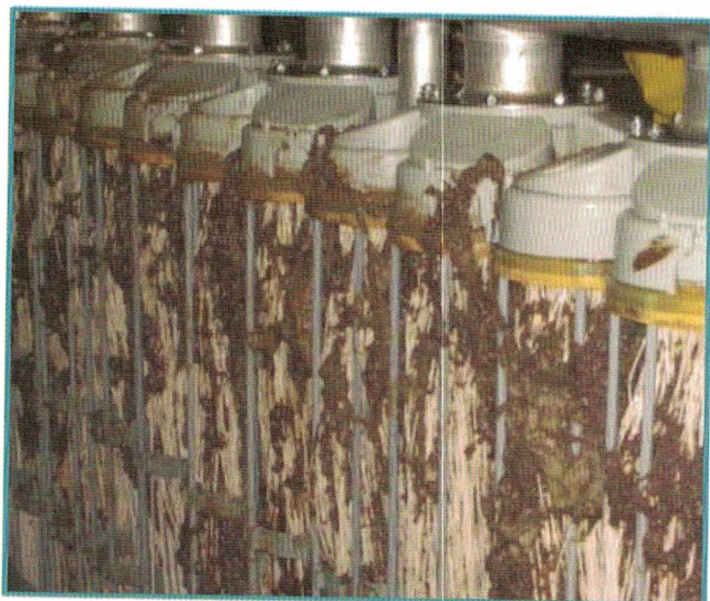
Figure 5. Debris fouling of tubular membranes
