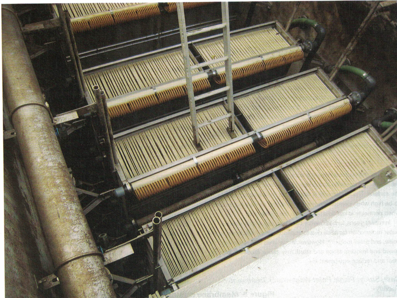
In the Pacific Northwest, 15 years of operational experience with membrane bioreactors has led to many lessons that can be applied to design and operation.
